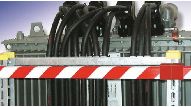
Barrier in a transformer station.
