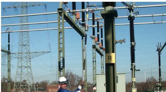
Use of an ASP distance voltage detector in an outdoor switching station
