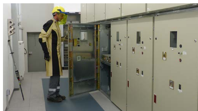
Switch room floor covered with insulating mat 50 kV.
