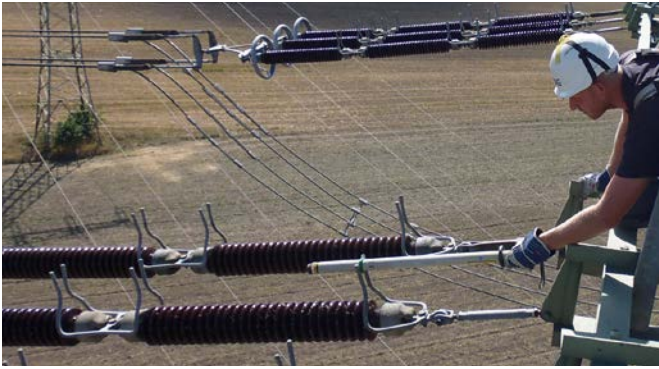
High-voltage indicator used on a 110 kV overhead line.
